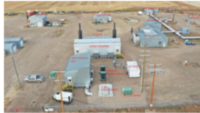
Figure 6: Journey Power Generation
